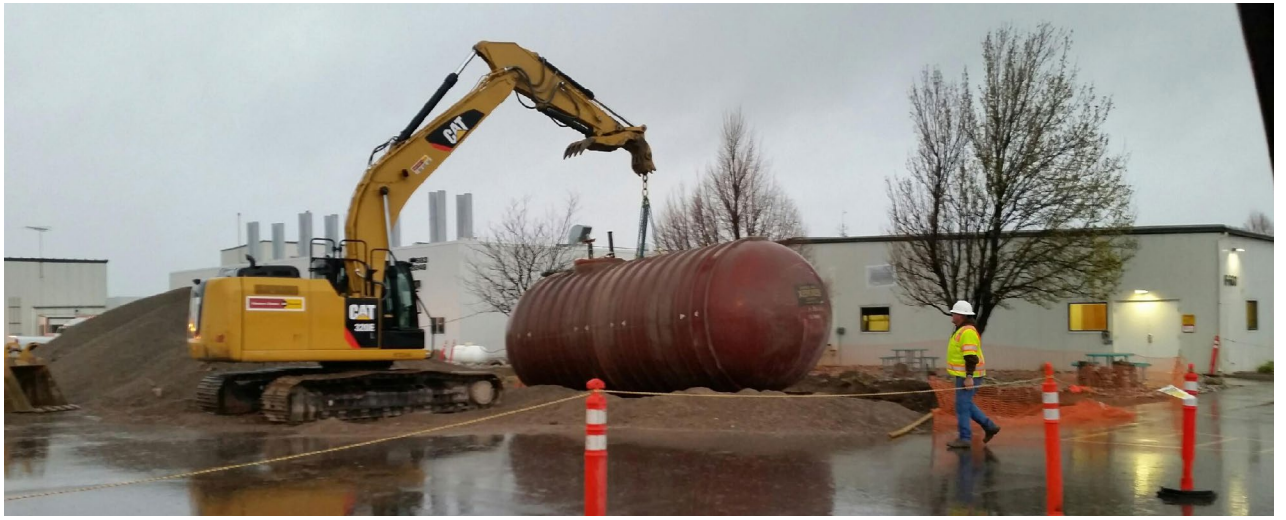
Removal of an old underground storage tank at the INL Research Center by NorthWind Construction, under the supervision of INL Construction Management, reduces leak risks from aging tanks and expanding EPA regulations.
