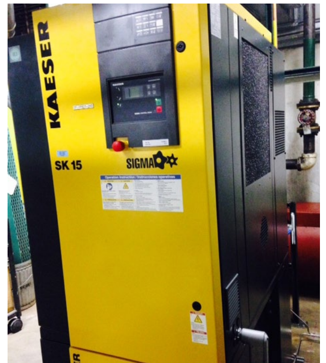
Efficient new air compressor for CFA-623
